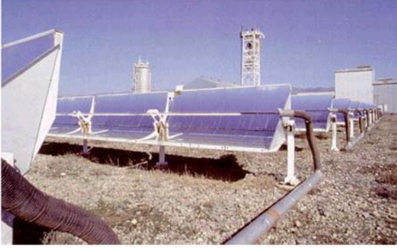
Fig. 1. The distributed solar collector field at PSA.
