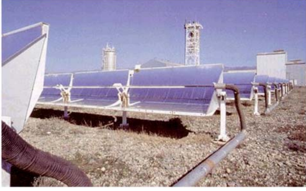
Fig. 3. The distributed solar collector field at PSA.
