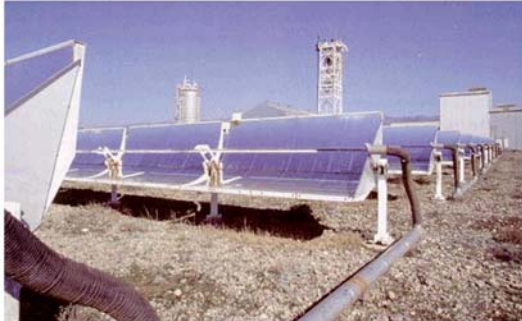
Fig. 3. The distributed solar collector field at PSA
